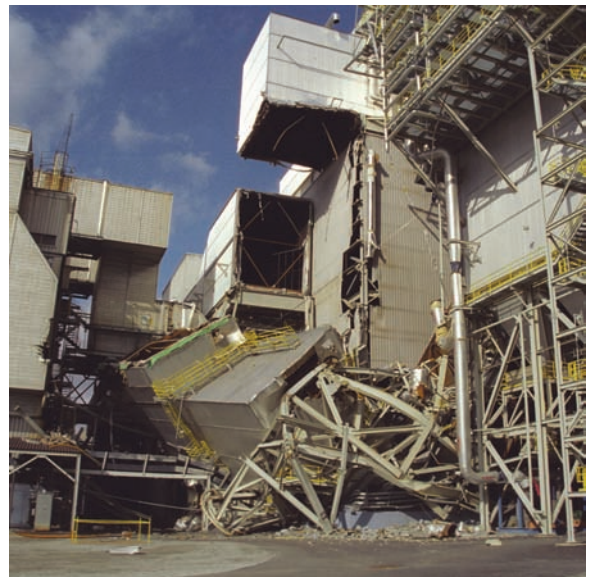
Power Plant Structural Collapse
