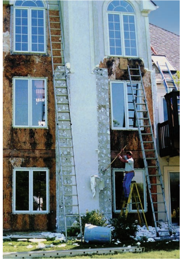
Mold growth and wood decay under barrier EIFS due to water infiltration
